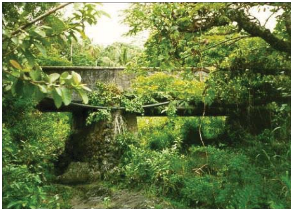
Figure 42. Papahawahawa Stream Bridge, a concrete beam and slab style bridge (Wilson Okamoto & Associates 2001)
