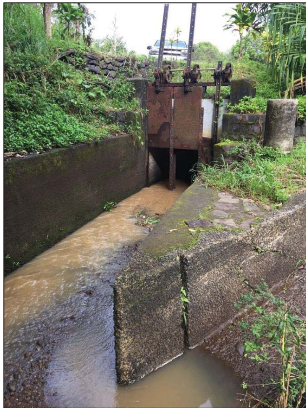
Figure 55. Control gate (Ha'ikū Ditch by Honopou Stream) (CSH 2018)
