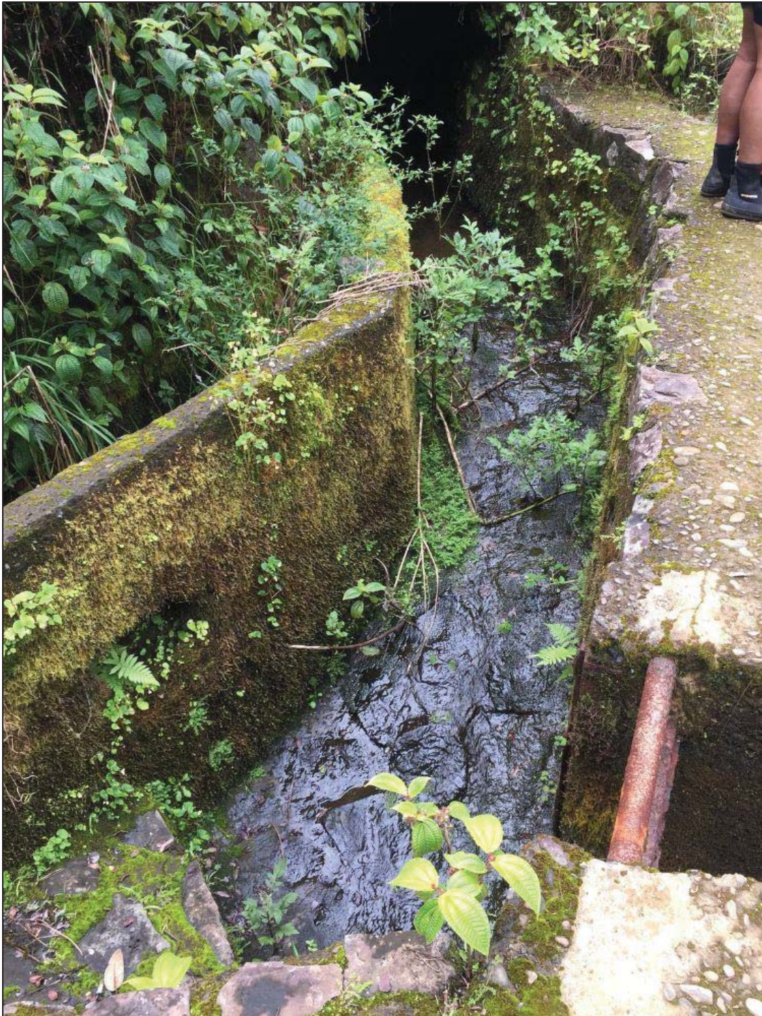
Figure 66. Waiohue control gate removed; intake blocked on other side (CSH 2018)
